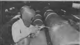
WELDERS, working beneath pier, joined pipe ends. WELDERS, trahando baxo pier, ta join pintonan di tabu.
